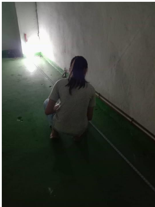
Figure 4.3.1.2 Testing at Electric Room The Sphere Mall Bangsar South, Kuala Lumpur
