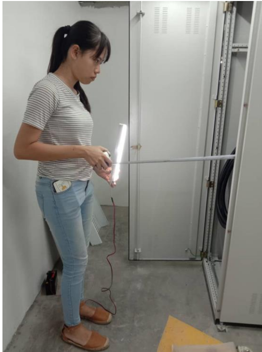
Figure 4.3.4.1 Testing at Electric Room NU Sentral, Kuala Lumpur
