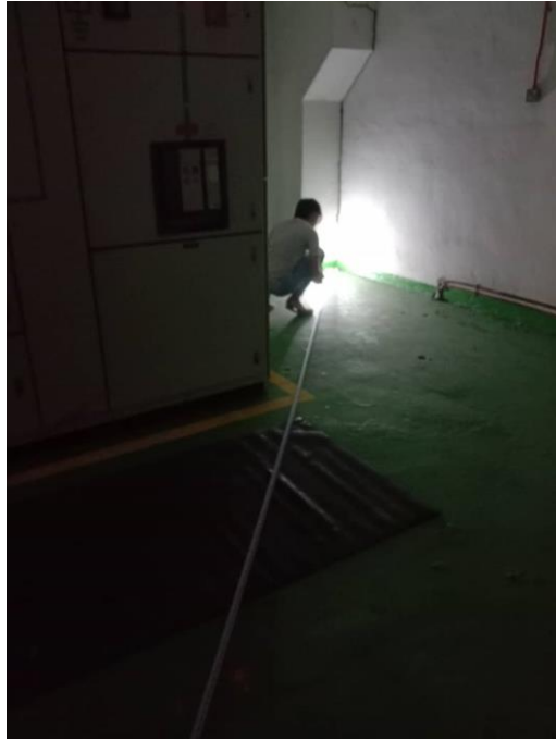
Figure 4.3.1.1 Testing at Electric Room The Sphere Mall Bangsar South, Kuala Lumpur
