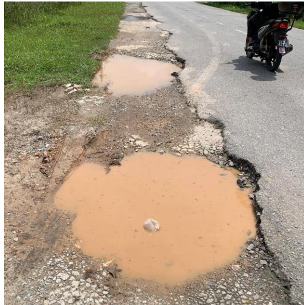
Figure 4.3.3. Road shoulder damaged with potholes and erosion
