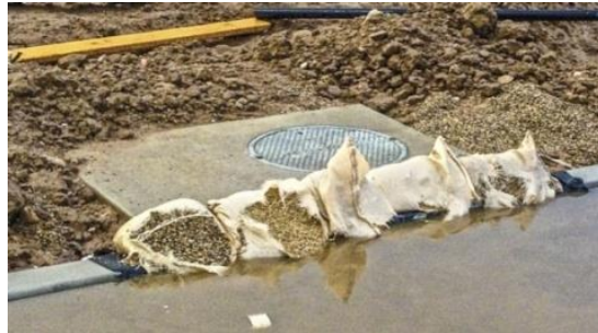
Figure 3: Sandbag that is broken after the flood.
