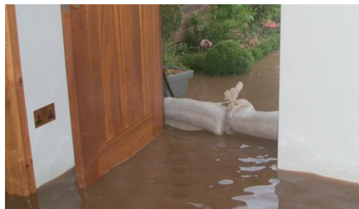
Figure 4: The sandbags cannot stop the water
