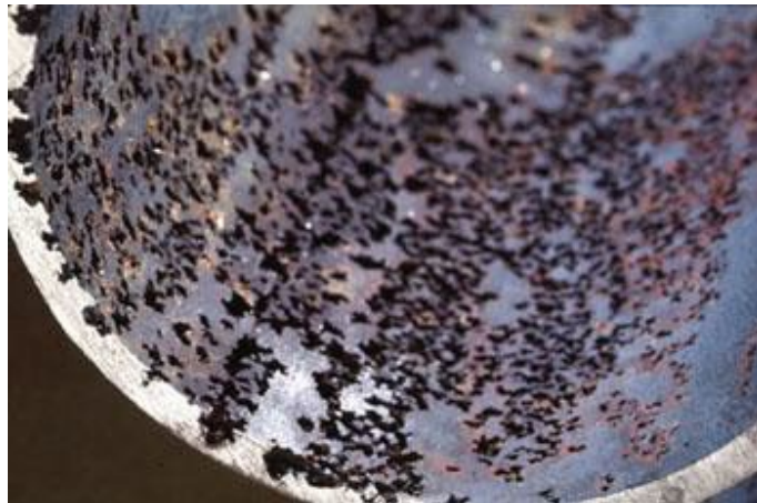
Figure 4.1: Corrosion in stainless steel pipe.
