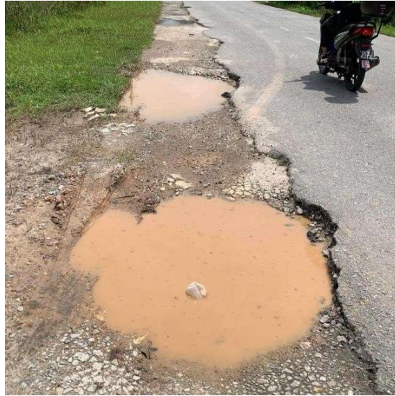
Figure 4.3.3. Road shoulder damaged with potholes and erosion
