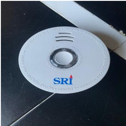
Figure 3.8 : SRI battery operated smoke sensor
